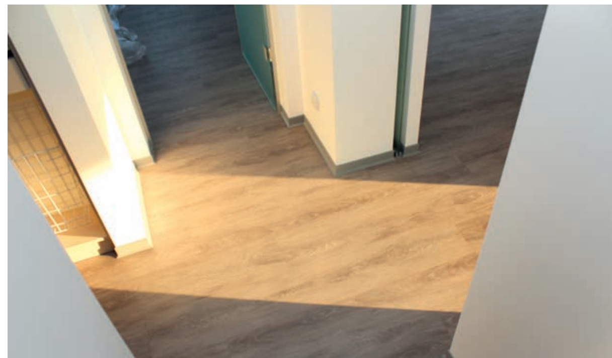
● Absence dilatace v podlaze
